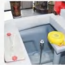
Large Opening Sewage Tank
