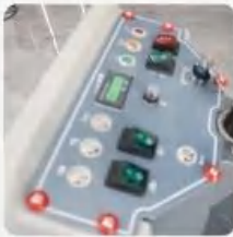
Simple Control Panel
